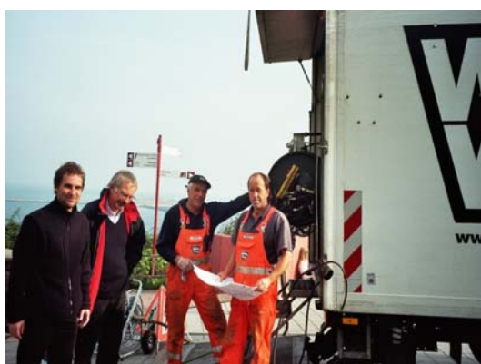
Herr Hagmeier (Bauamt Helgoland), Herr Losch (Ing.-Büro Losch & Partner), Herr Gärtner (WeVo), Herr Morgenthal (WeVo)
